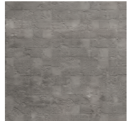
RIPPED-OUT | ARRANCADO - PK16905RT [R12C]
